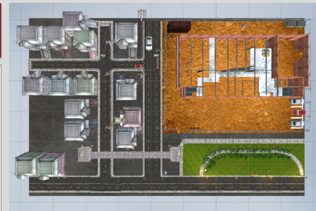
An aerial view of the construction site and surrounding environment PC: Maylin Martinez
